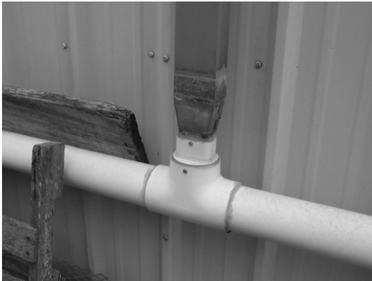
Figure 10.6. The transition in the downspout to conveyance piping is causing a reduction in flow.
