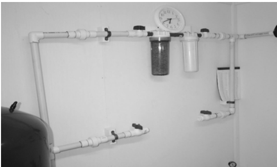
Figure 16.15. Isolation valves allow re-routing of water, as well as removal and replacement of component.
