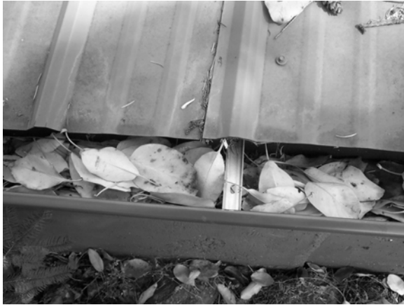
Figure 17.2. Debris lodged in a gutter can block the downspout screen and result in a flooded gutter.
