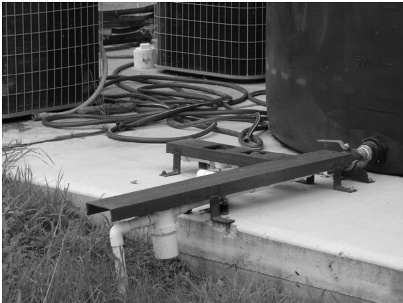
Figure 13.9. Valves and piping are protected.
