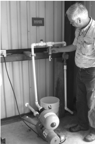
Figure 16.13. An accessible filter is easy to maintain and replace.
