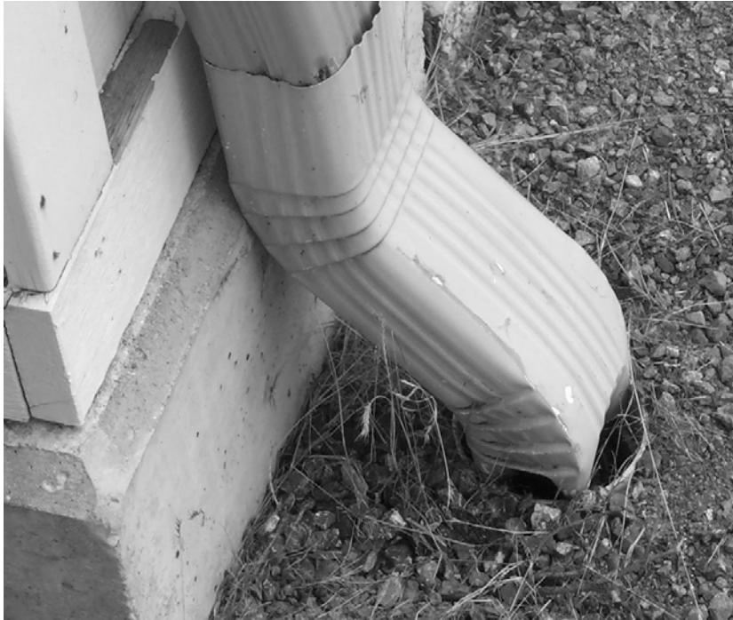
Figure 10.7 A ground-level transition facilitates contamination from surface runoff.
