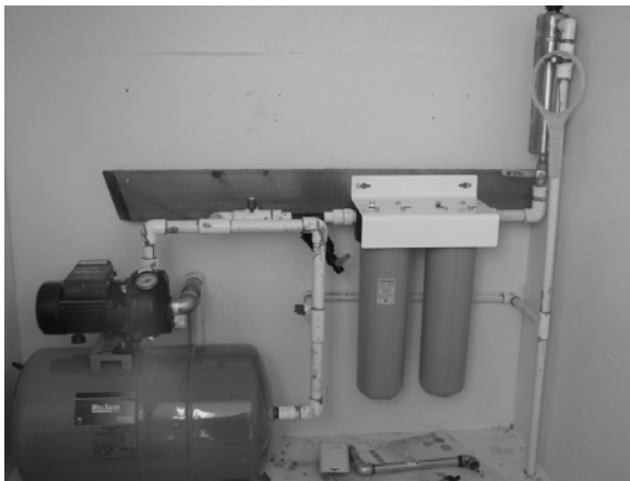
Figure 16.17 The pump, pressure tank, filters, and UV device are all hard-plumbed making maintenance and replacement of components difficult.
