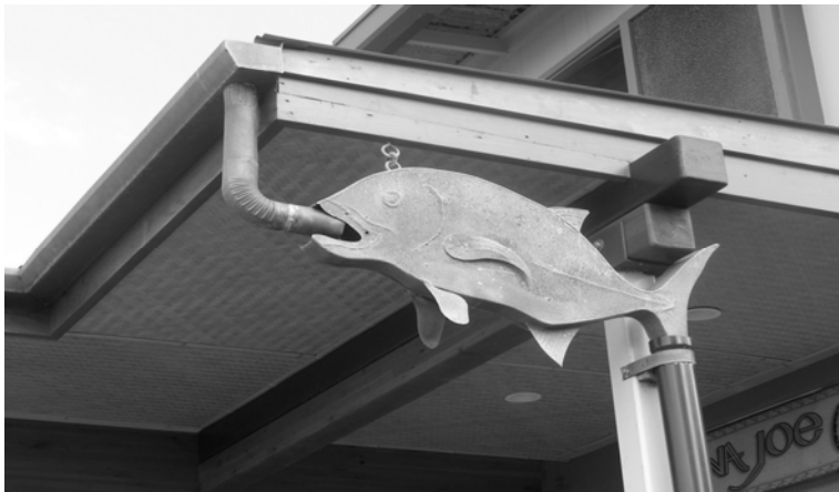
Figure 10.5. A downspout transition is covered by an aesthetically appealing design made to look like a fish.
