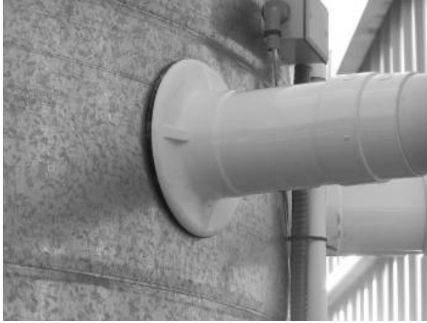
Figure 12.4. Inlet and outlet.
