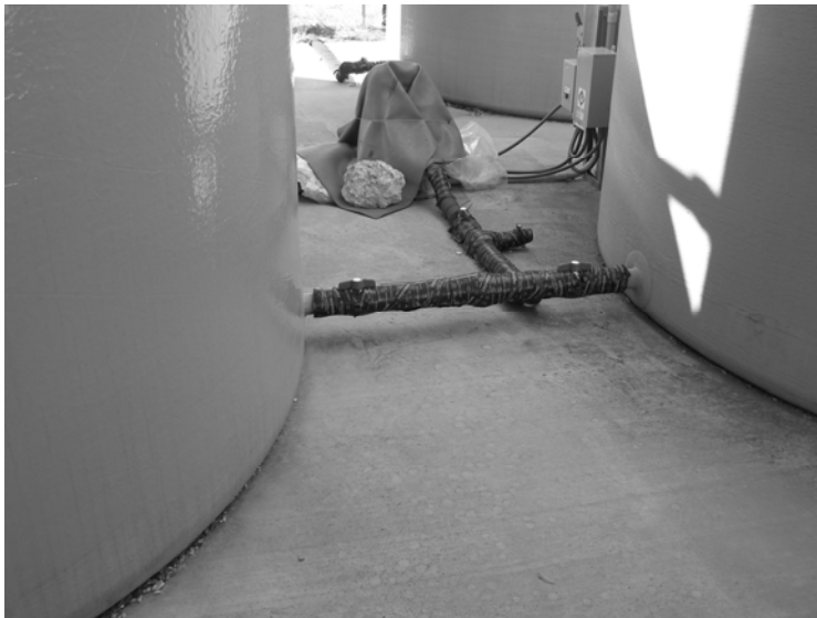
Figure 13.6. Isolation valves between tanks.
