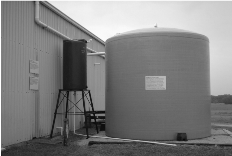
Figure 11.11. Roof washer on stand located adjacent to an above ground tank.
