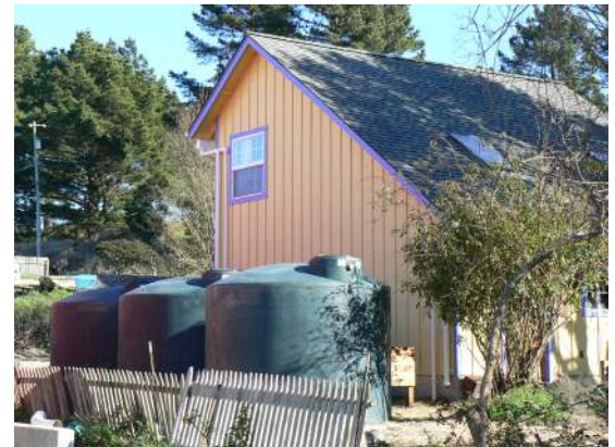
TOP TO BOTTOM: Gilardi Ranch catchment installation; Bodega Volunteer Fire Department storage tank; private residence roofwater harvesting system. Photos courtesy of Lauren Hammack, Prunuske Chatham, Inc. and John Green, Gold Ridge Resource Conservation District.
